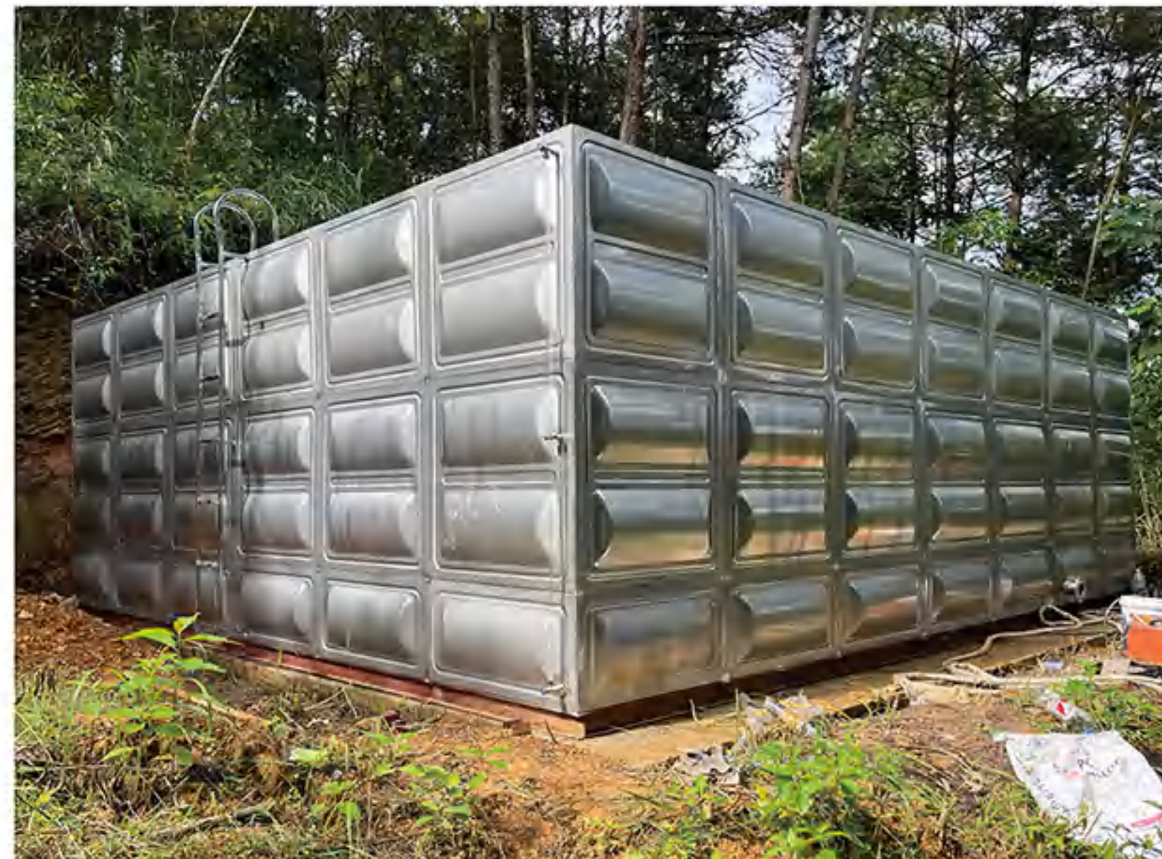
120 tons water tank in Cote d'Ivoire, Africa
