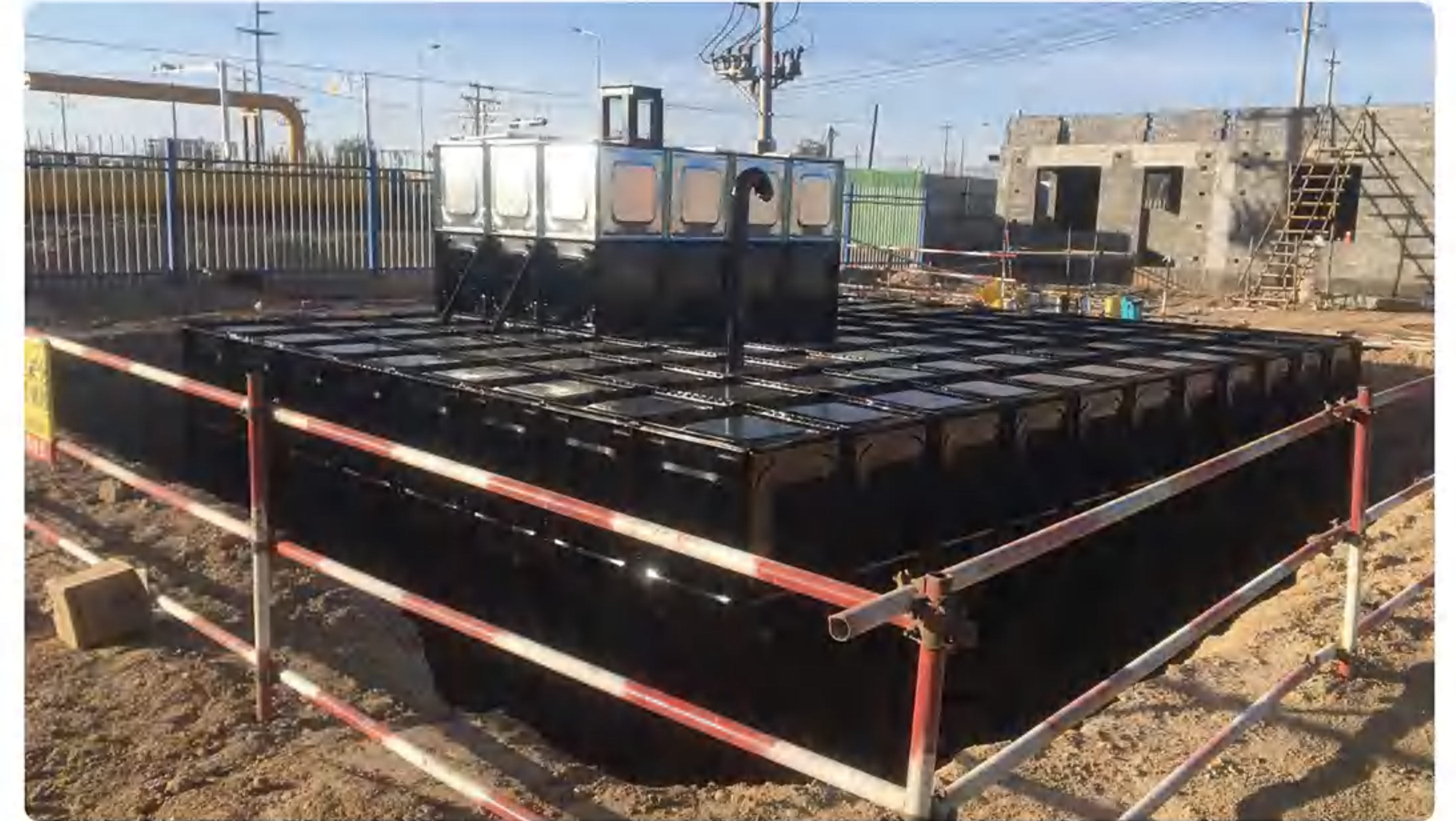
Guangxi Ruihong Construction Group Co., Ltd. 350 tons water tank
