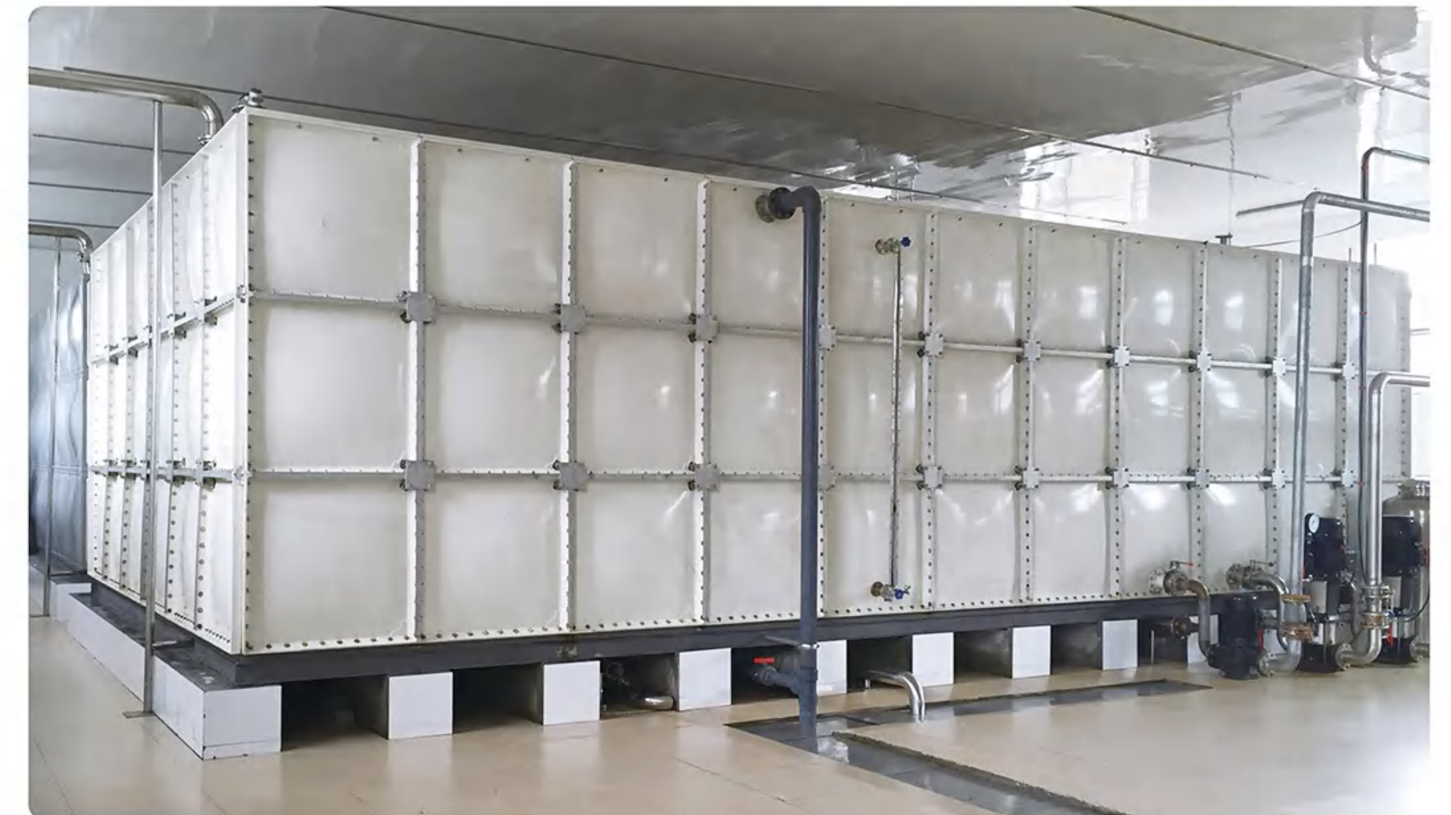
Jiangxi Longxiang Lithium Battery Co., Ltd. 200 tons water tank
