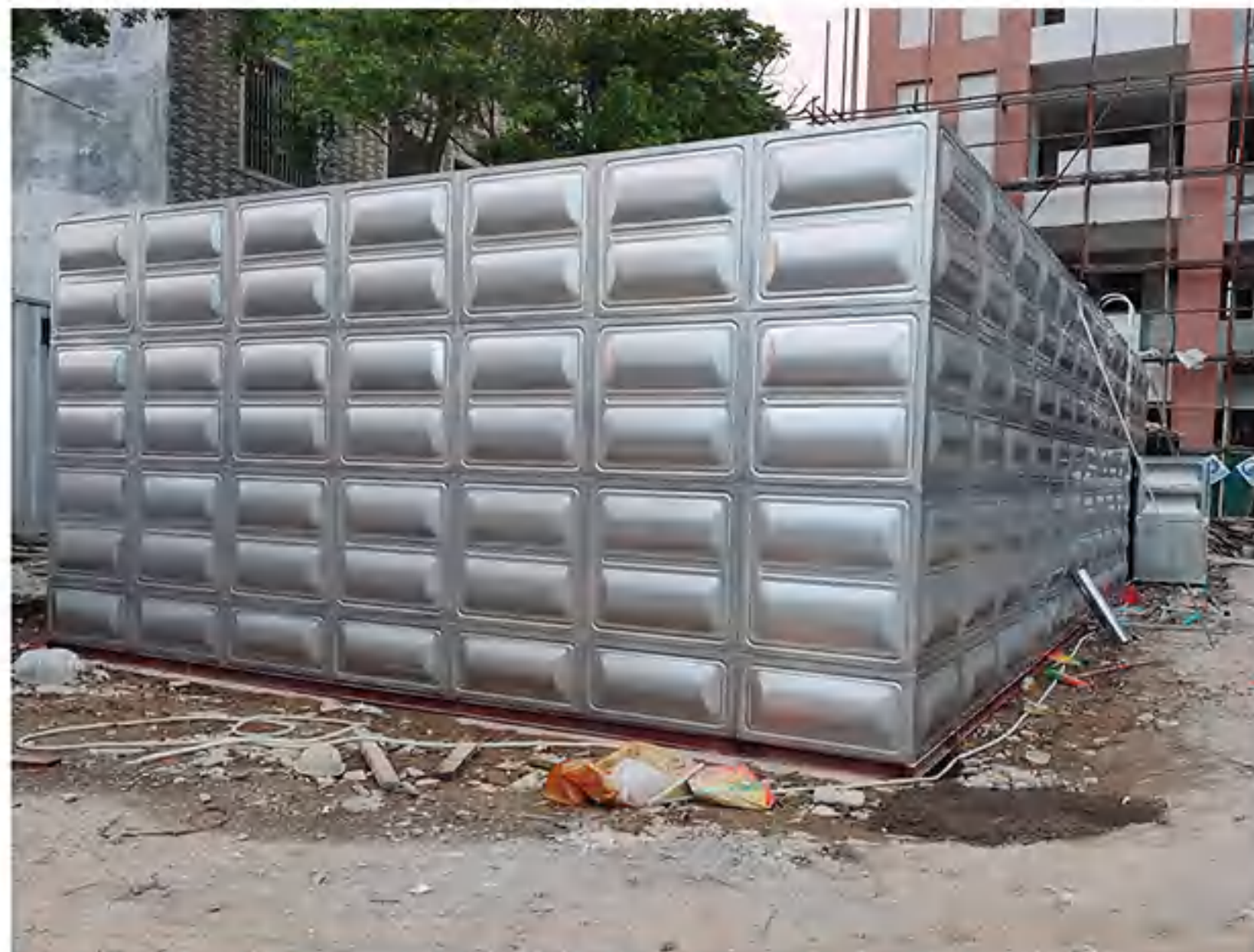
240 ton water tank with pump room in Heyuan City, Guangdong Province
