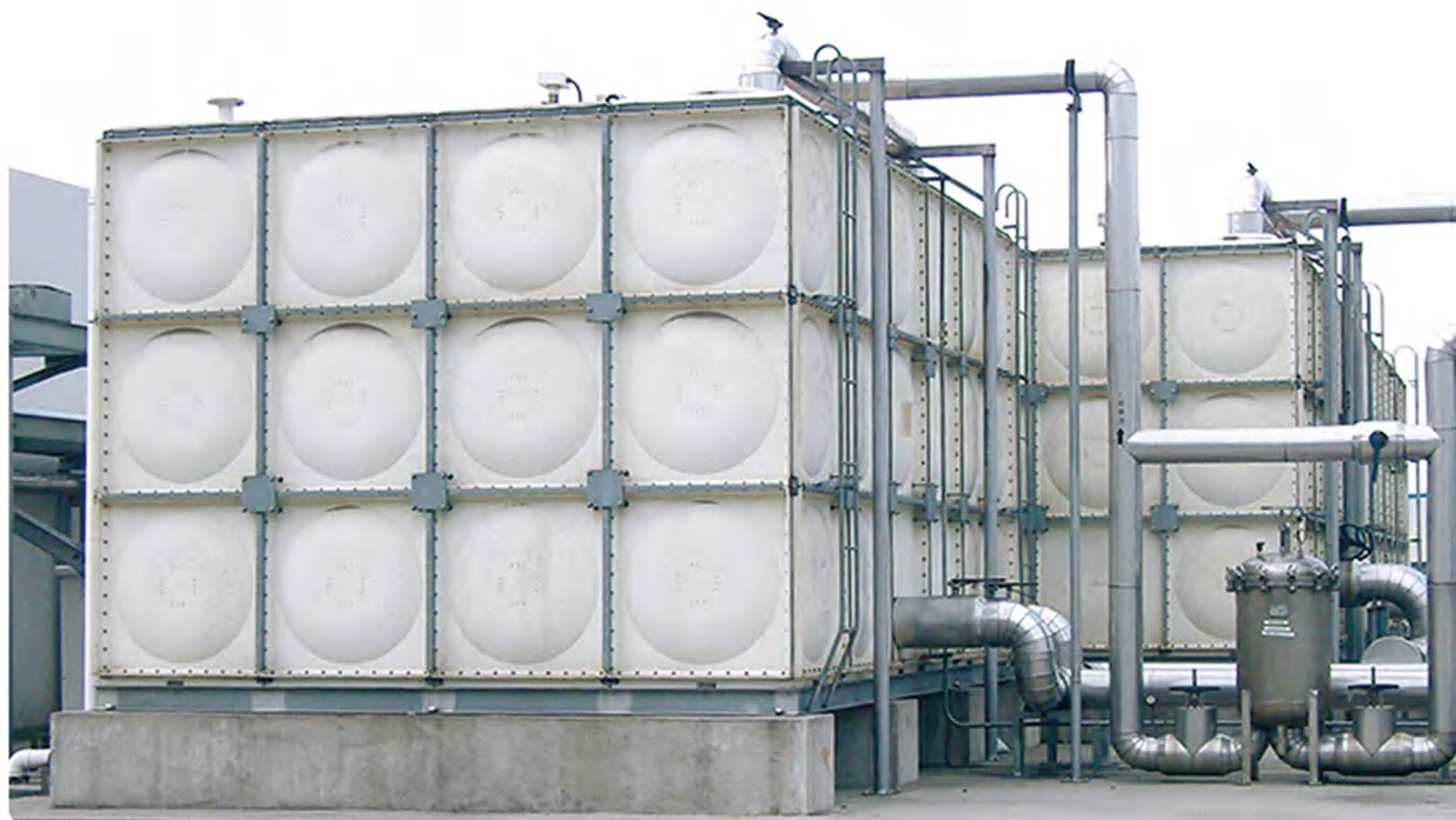
Cambodia Poipet project 150 tons water tank
