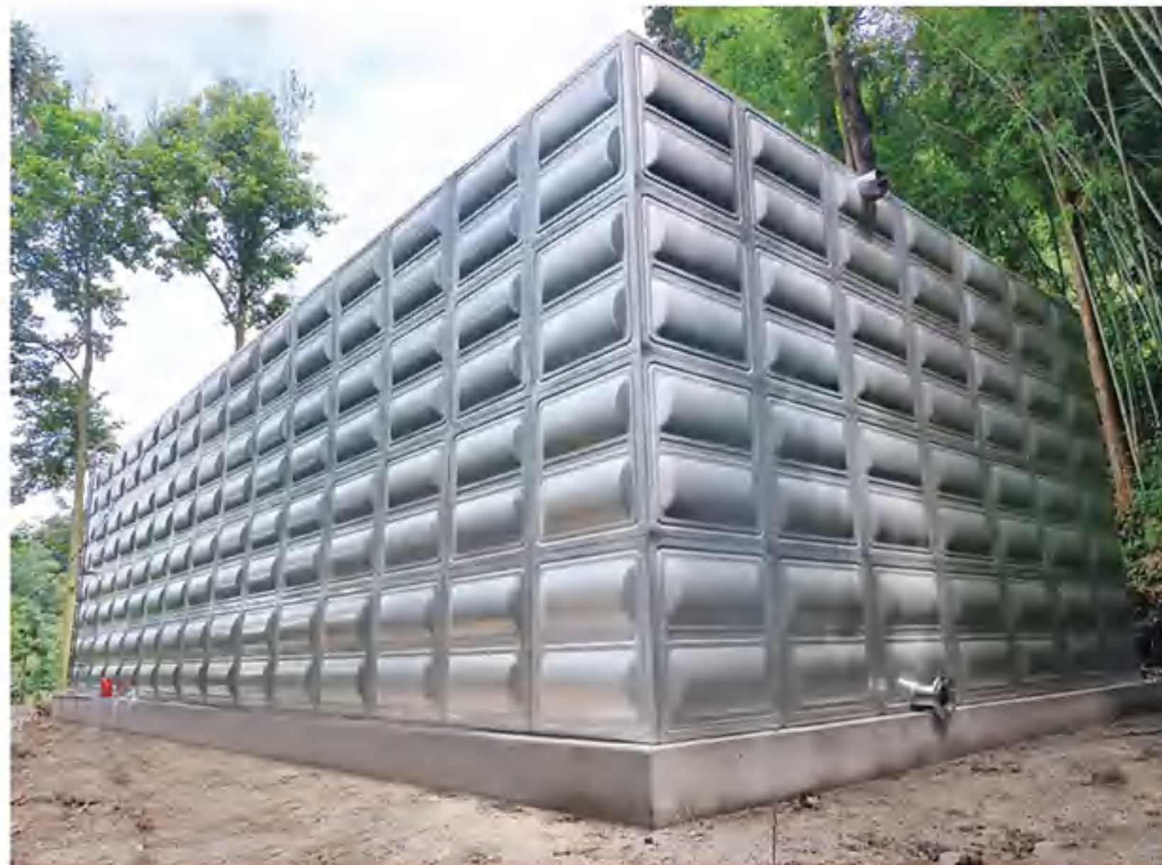
480-ton water tank in Shuigougu Village, Kayin State, Myanmar
