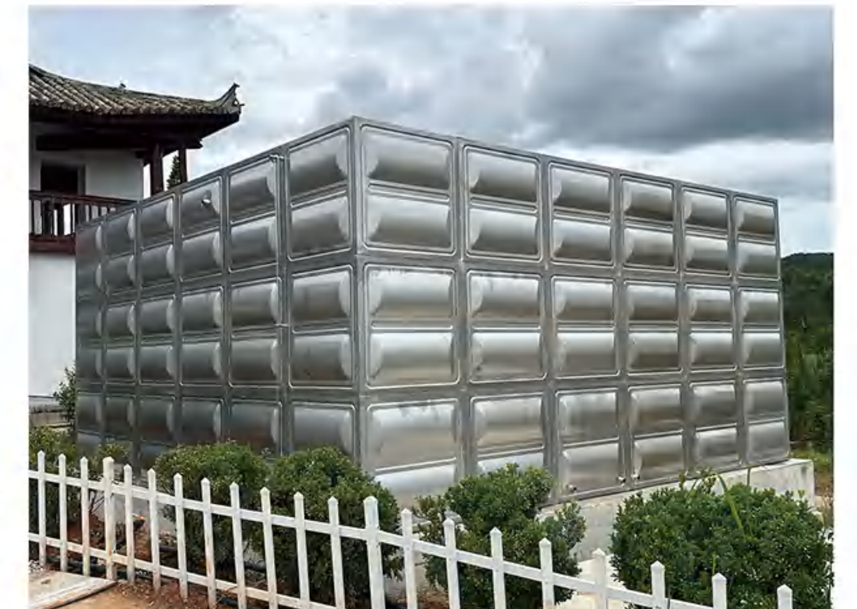
108 ton water tank in Lincang City, Yunnan Province
