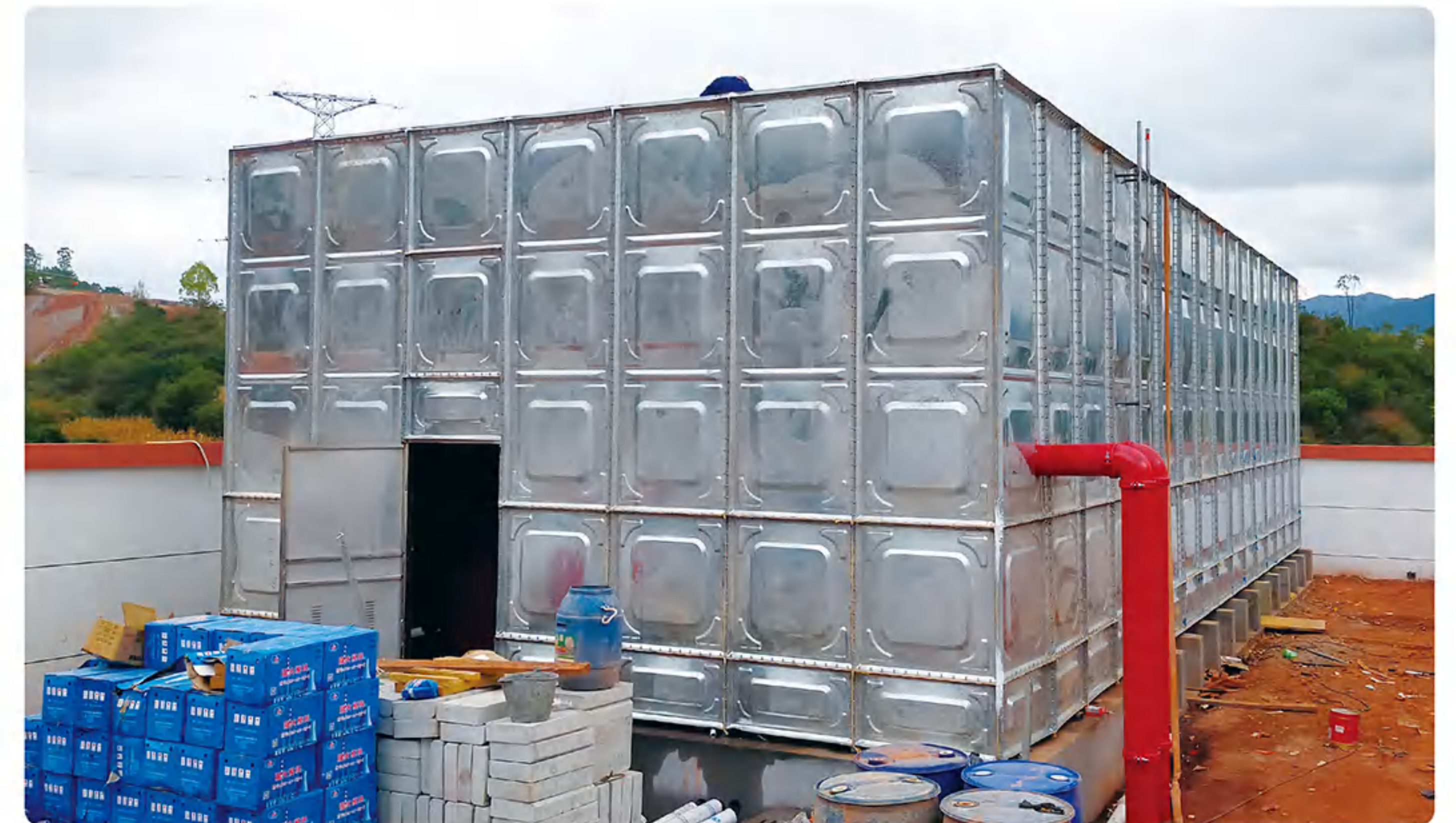
Suzhou Jiazhai Yishu Architectural Decoration Design Engineering Co., Ltd. 600 tons water tank
