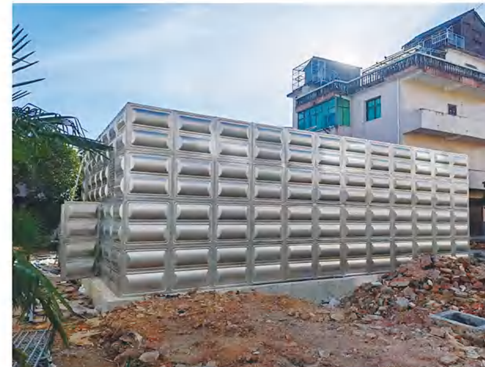
420 ton water tank with pump house in Nancheng County, Jiangxi Province
