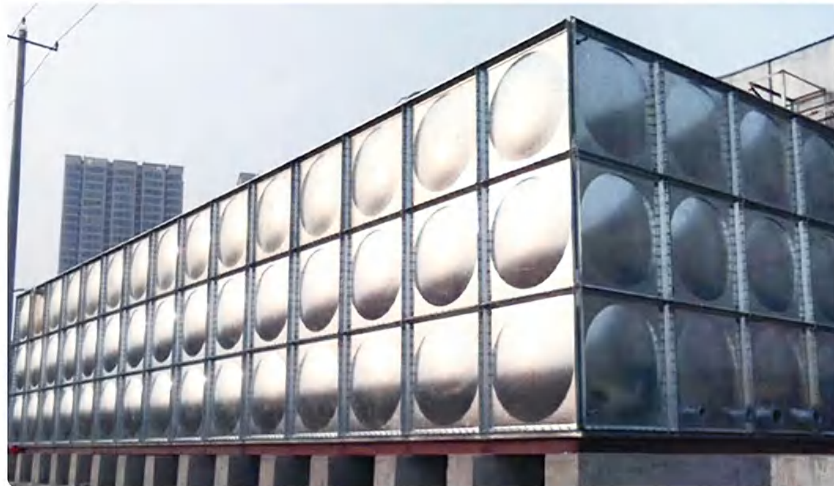
Shenzhen Hefengjiada Technology Co., Ltd. 280 tons water tank
