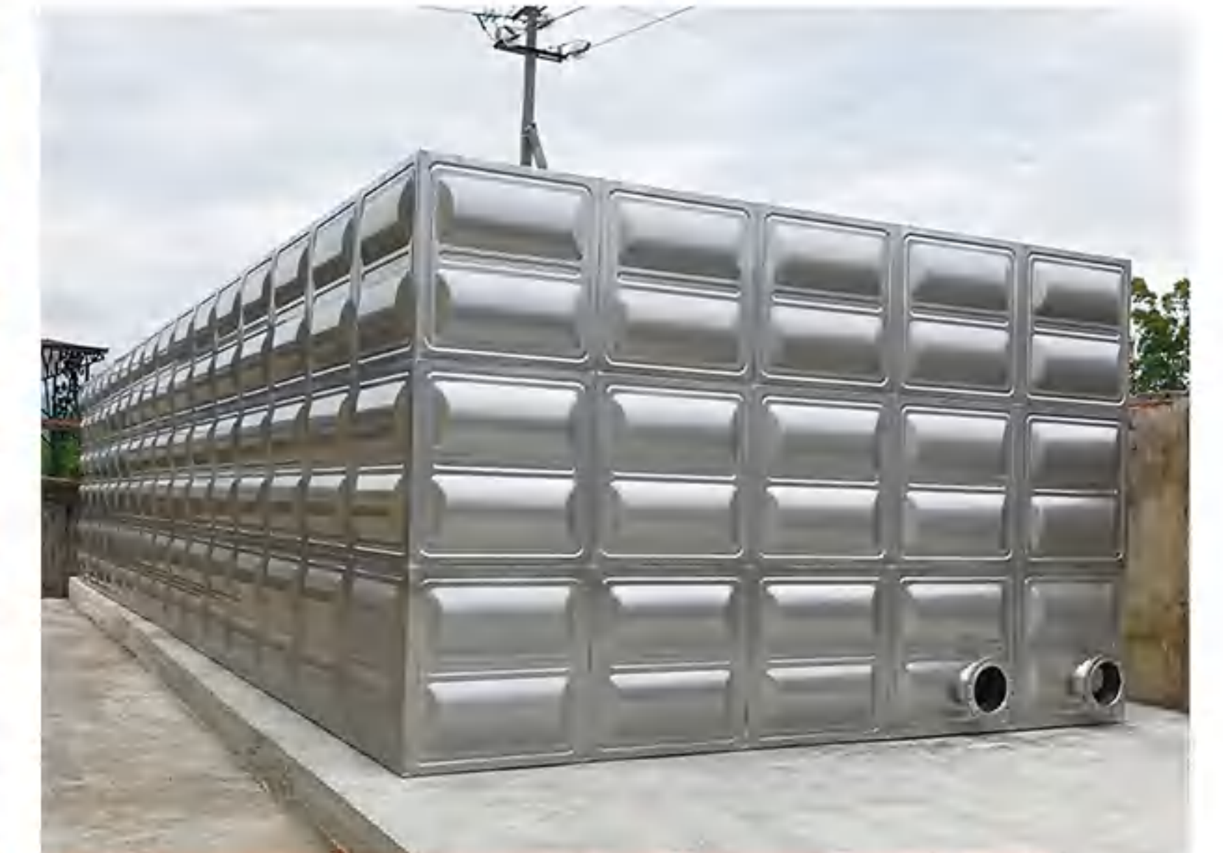
240 tons water tank in Yuanling County, Huaihua City, Hunan Province
