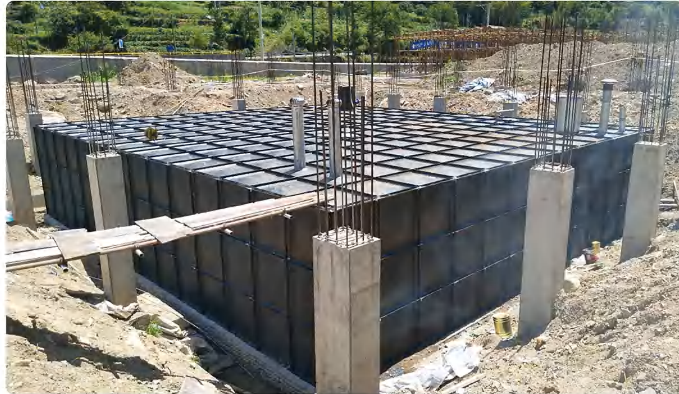
Anhui Yuhong Construction Engineering Co., Ltd. 600 tons water tank
