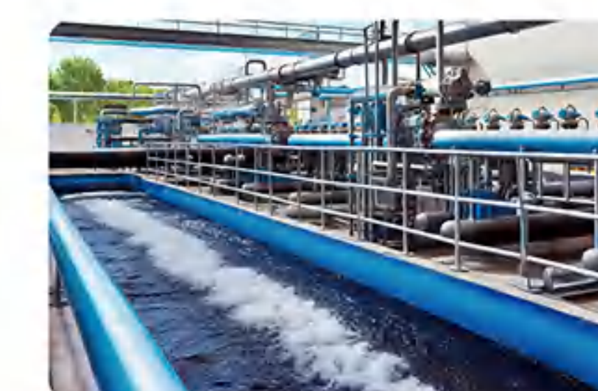
Waterworks Pumping Station
