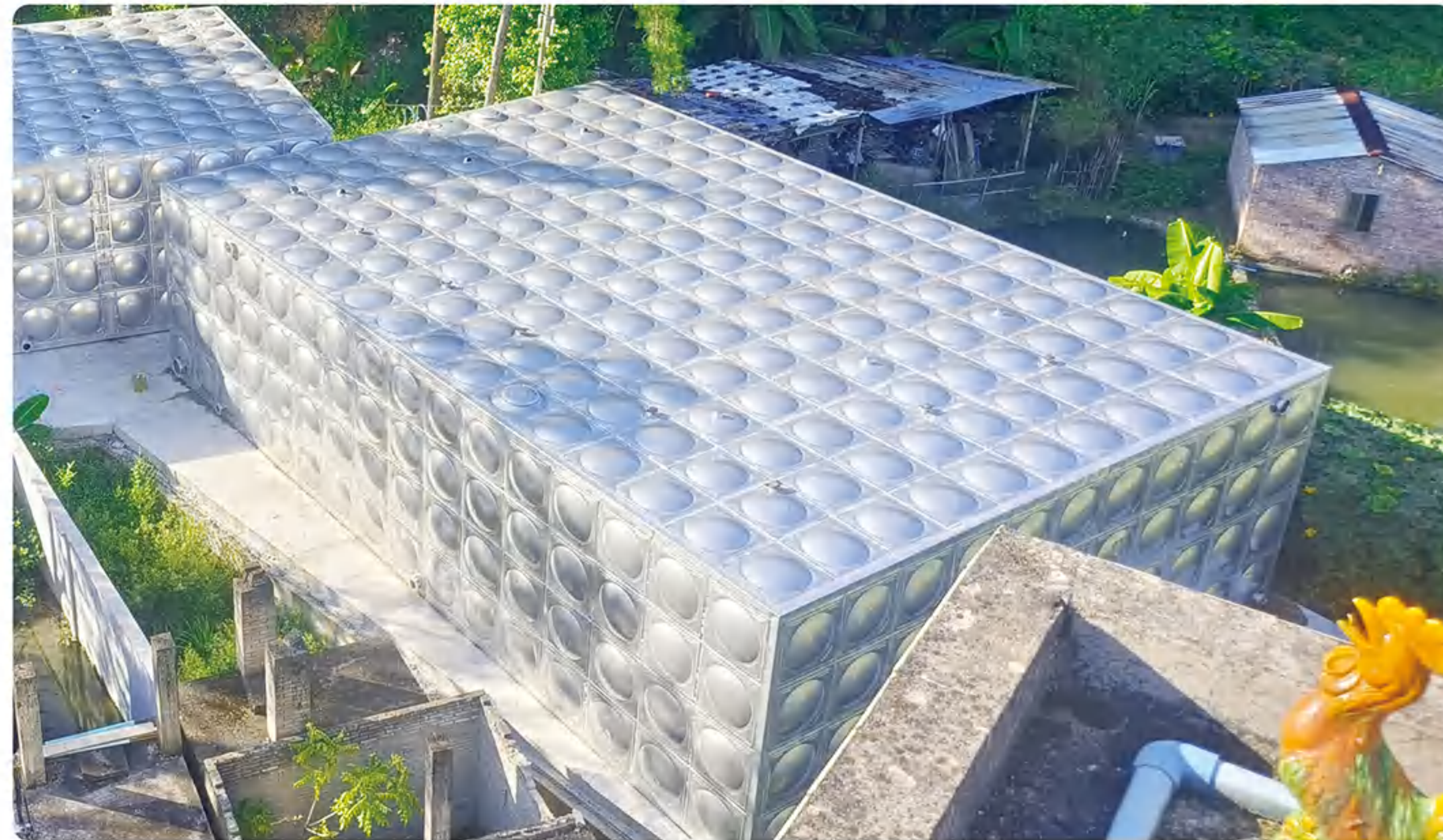
CENXI YANGSHENG MINING CO., LTD. 1200 TONS WATER TANK
