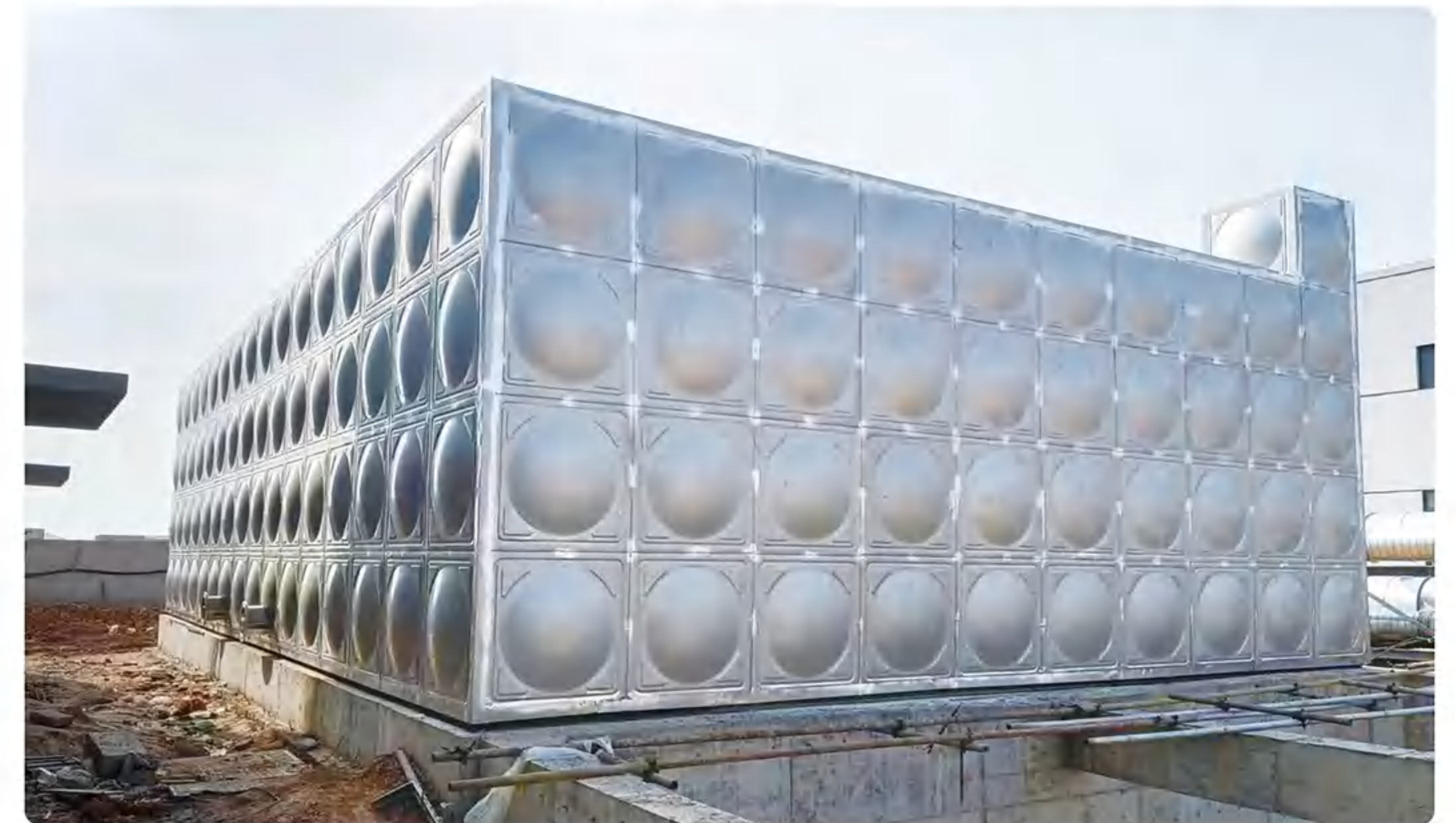
DONGGUAN CHENGHUI CONSTRUCTION ENGINEERING CO., LTD. 760 TONS WATER TANK
